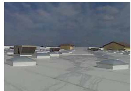
A new "Cool Roof" atop a Wal-Mart Supercenter in Orlando reflects solar heat away from the building, reducing cooling costs.
